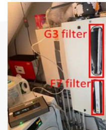
Ventilation unit with heat recovery in all 4 dwellings
