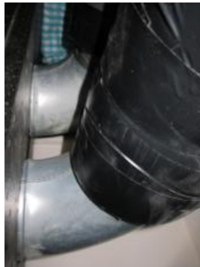
Figure 8 –Passive House MVHR Insulation
