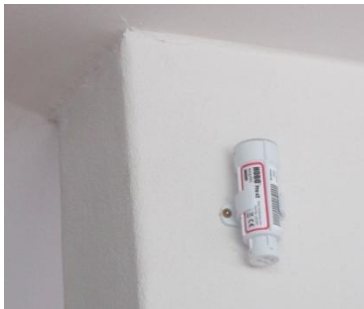
Figure 5 Installation of data logger (room sensor) to detect the indoor climate
