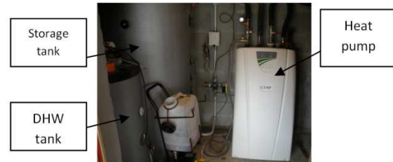
Figure 3. Heat pump and storage tank.
