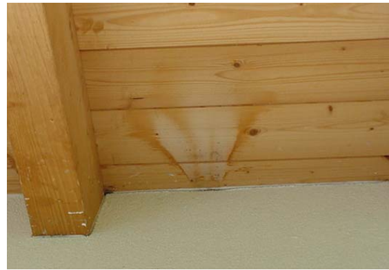
Figure 16: Exfiltrating warm and moist room air condenses at the roof panels and clearly discolors the wood.
