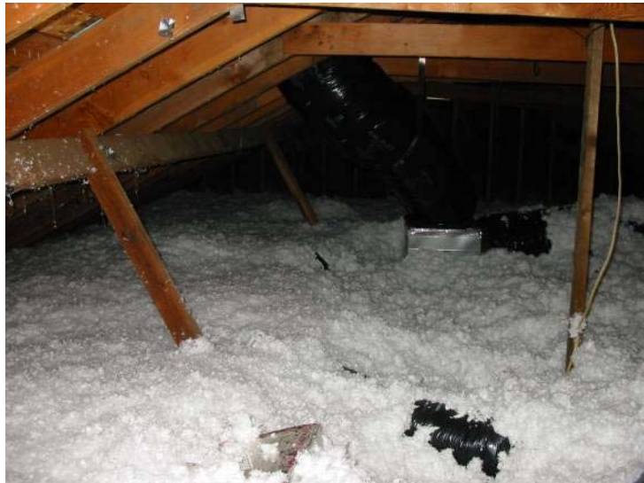
Figure 4. New flex ducts in attic covered by additional blown-in insulation.
