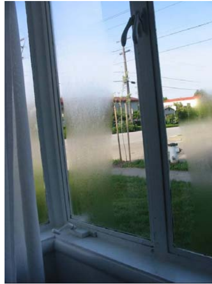
Less extreme is this typical condensation in single pane windows
