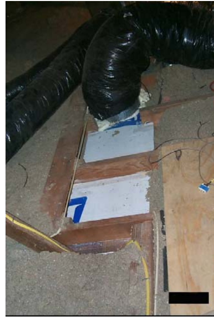
Envelope sealing: Often there are large building cavities or chases that are open to outside via attics, crawlspaces or garages. This is an example of a sealed chase viewed from the attic. The large white rectangles are duct board insulation that has been used to block off large open areas
