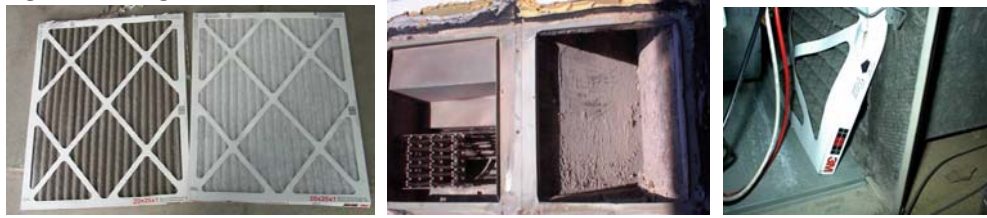
These illustrations show dirty and clean pleated filters, a very dirty coil that had been exposed to unfiltered air and a poorly installed filter that leads to filter bypass and most of the air flowing through this system would be unfiltered.
