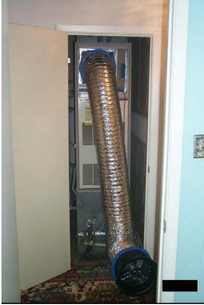
Pressure matching using an auxiliary fan and flowmeter
