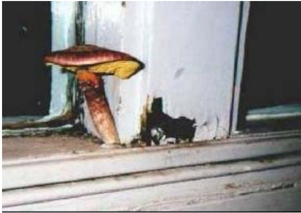
Extreme moisture problems lead to wood rot and fungal growth
