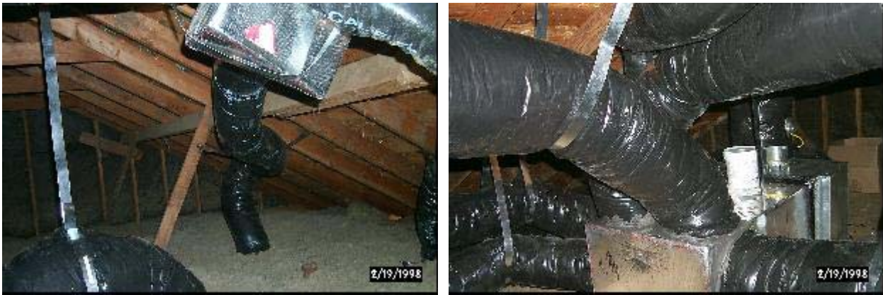
Figure 12. Initial installation of ductwork hanging from ceiling of attic [right shows smooth bend out of plenum].
