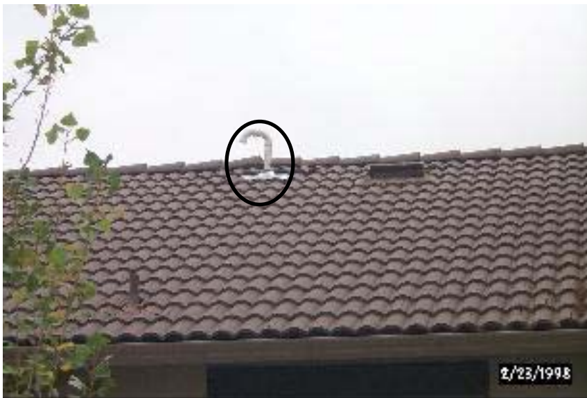
Figure 9. Installed roof mounted furnace flue pipe.
