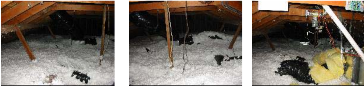
Figure 15. Attic floor with flexible ducts and additional blown-in insulation over ducts. The yellow material is fiberglass wrap insulation.
