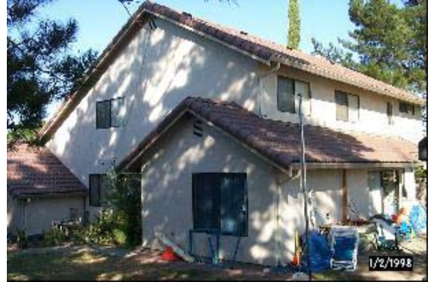
Figure 2(b). Exterior side view of Concord test residence showing gable attic vents and existing outside AC condenser unit placement [lower left].
