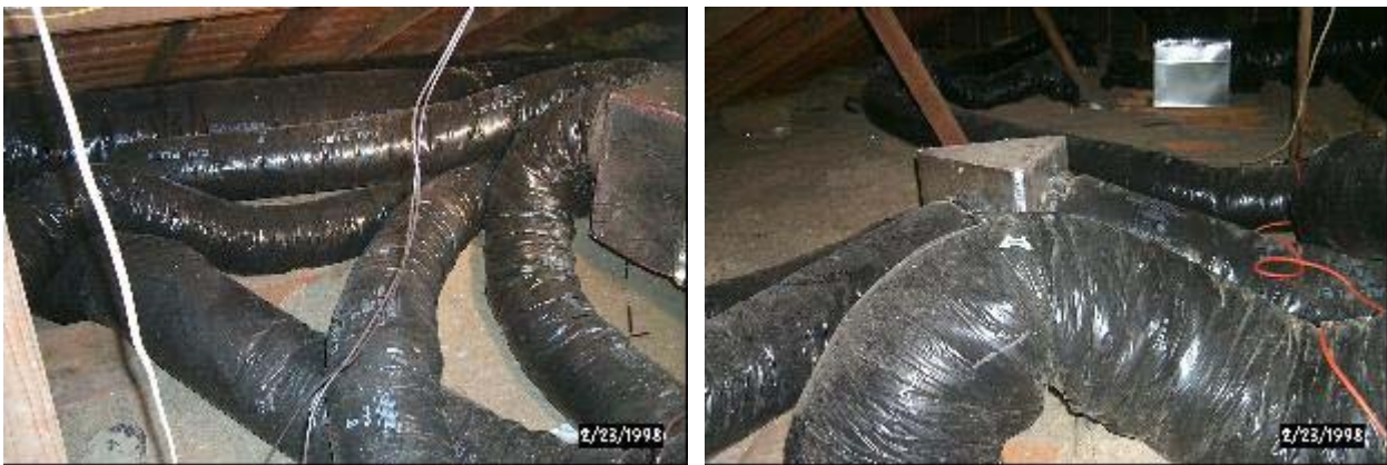
Figure 14. Second and final installed retrofit of ductwork after being moved to attic floor and before adding insulation showing tight bends.
