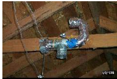
Photo B.7. Attic air aspirated temperature and relative humidity sensors located near attic ceiling.
