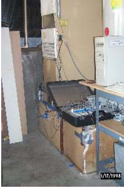
Photo B1. Data acquisition equipment in garage with existing furnace in background.
