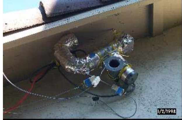
Photo B.2. Outdoor air aspirated temperature and relative humidity sensors located under roof eave.
