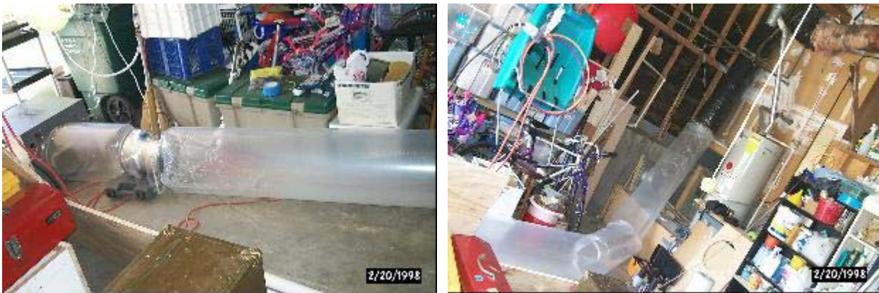
Figure 17. Aerosol apparatus for duct sealing in garage.
