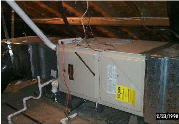
Figure 7(a). New cooling and heating equipment on attic floor [right to left: return plenum, air filter, air handler, furnace, cooling coil and supply plenum].
