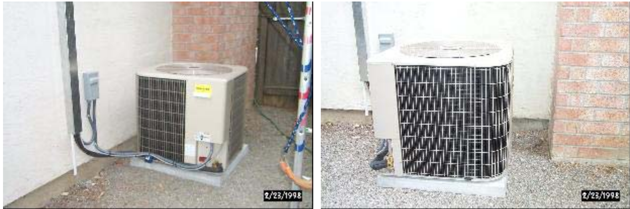
Figure 8. New AC condensing unit on shaded side of house.
