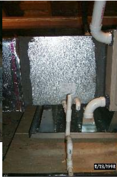
Figure 7(b). New cooling coil with condensate drains and top of furnace with combustion air intake and exhaust.
