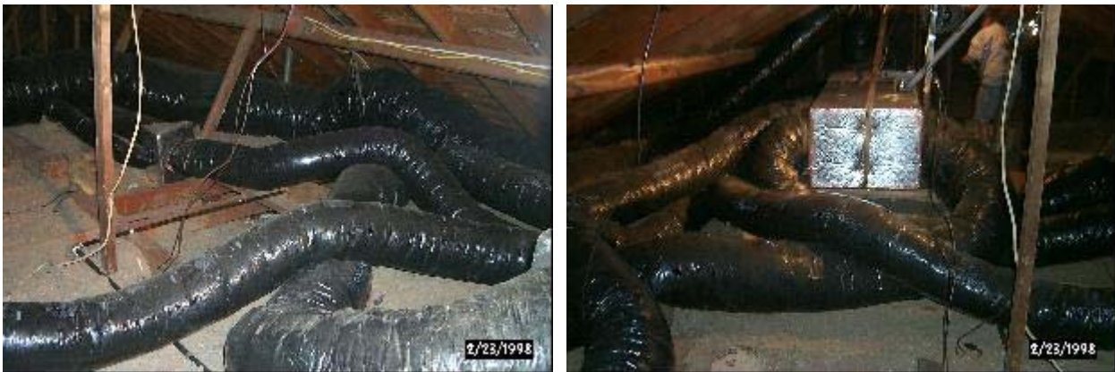
Figure 13. Second and final installed retrofit of ductwork after being moved to attic floor and before adding insulation.
