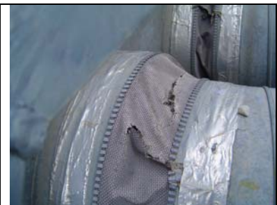
Picture 3: Leakages, ductwork
