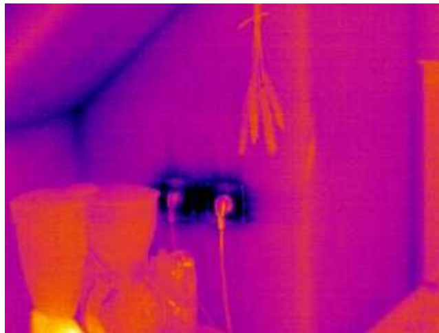
Figure 1. Photograph with IR-camera of electrical plugs. The building was depressurized with a blower-door.
