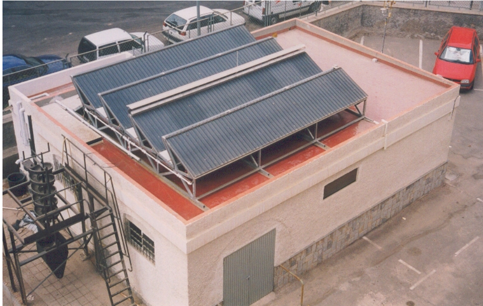
Solar roof erected at the Scholl of Engineers in the Polytechnic University of Cartagena (Spain)
