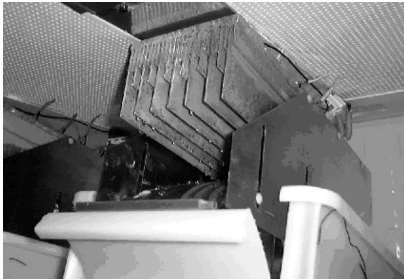
Figure 3 A condensing unit in operation
