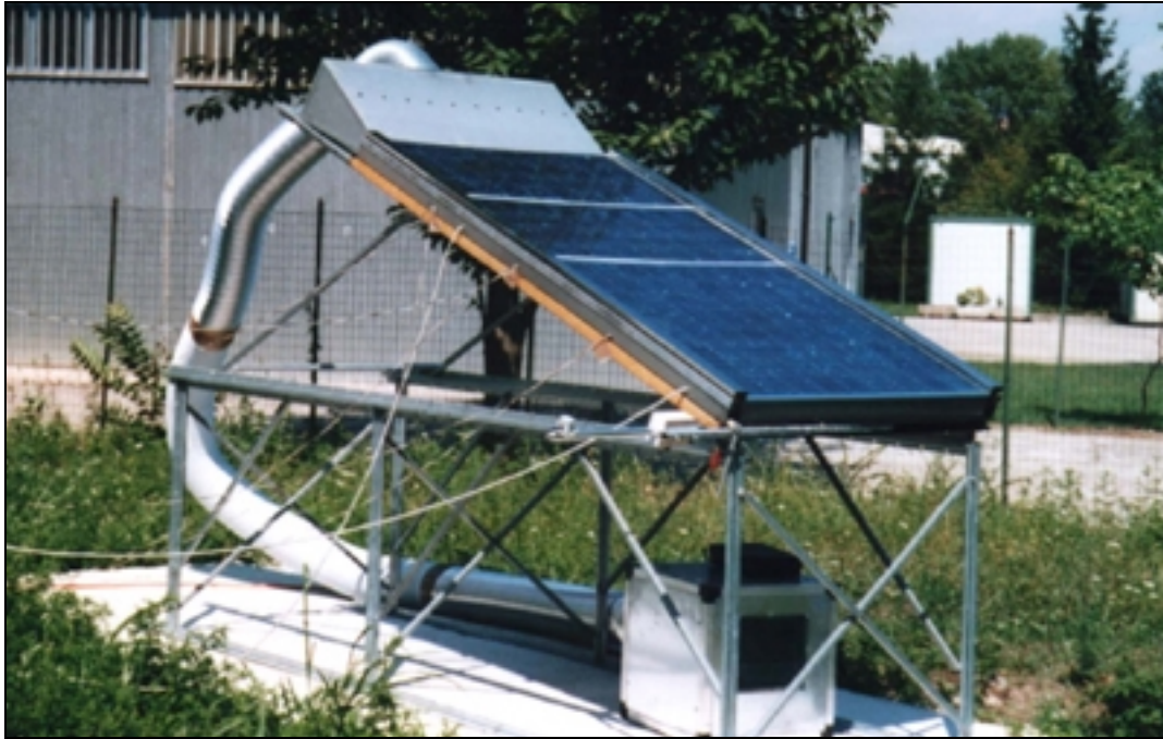
Figure 1: Test proto-type installation
