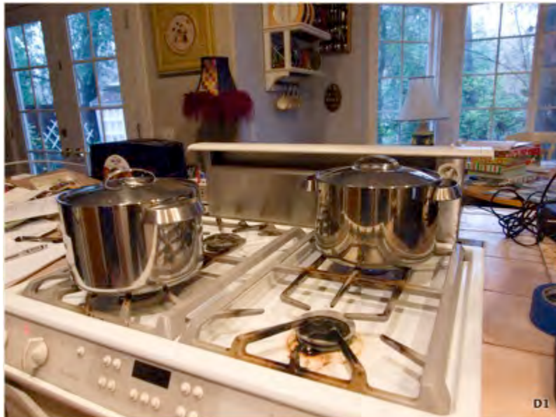
Figure 2. Downdraft exhaust system D1.
