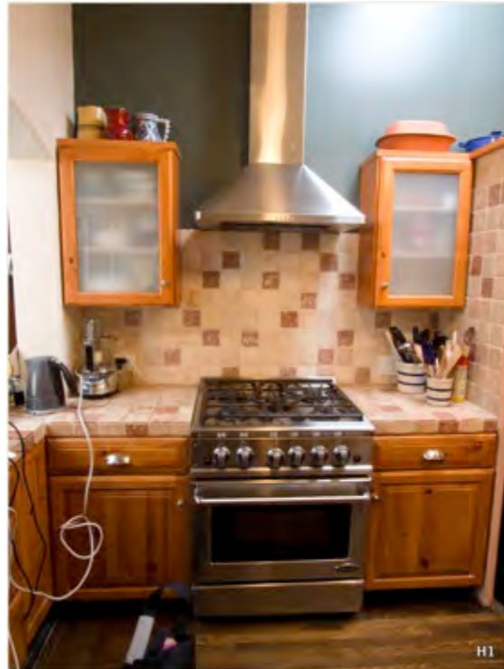
Figure 29. Exhaust System H1, placement in kitchen.
