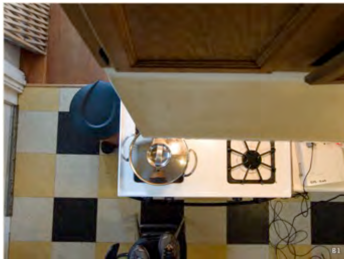
Figure 40. Exhaust System B1; top view showing incomplete coverage of cooktop.
