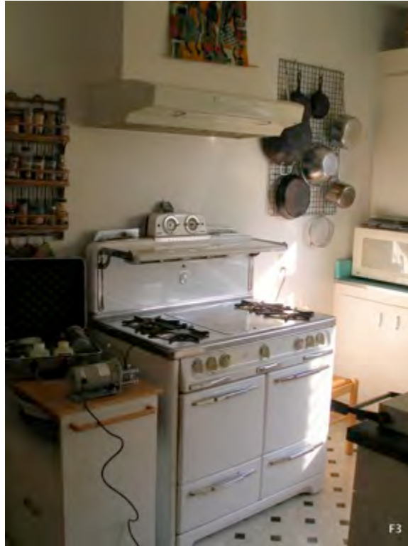
Figure 18. Exhaust system F3, location in kitchen.
