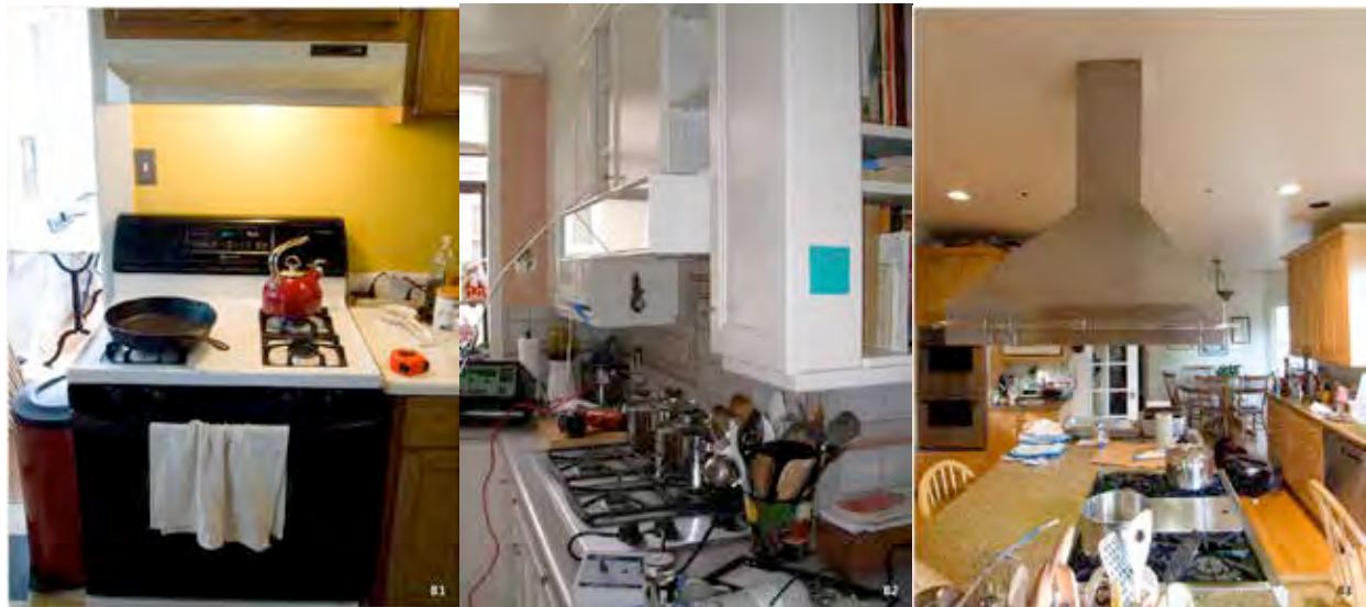
Figure 6. Exhaust systems with open capture hoods B1–B3
