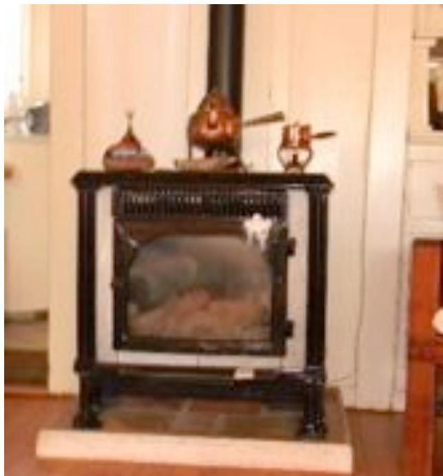
Figure 3.9 A picture of the gas fireplace at Site 1405, which has been identified as the cause for the elevated CO levels measured at the home.
