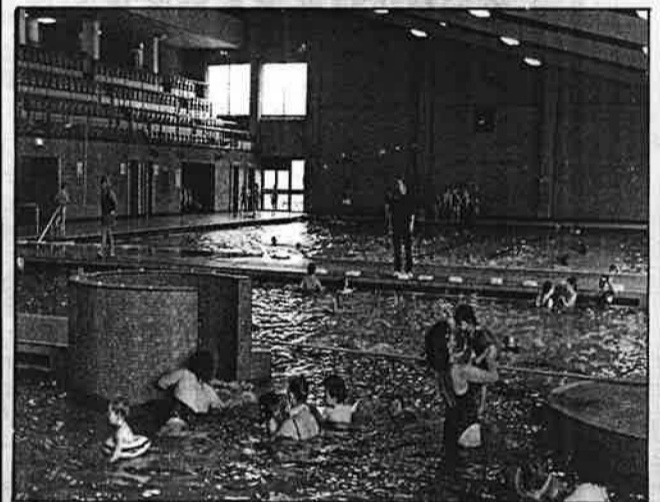
Replacing an eight-year-old steel-framed air-handling unit at Macclesfield Leisure Centre is an AAF unit, with a frame of Modar composite material, that will not corrode in the harsh chlorine atmosphere.
