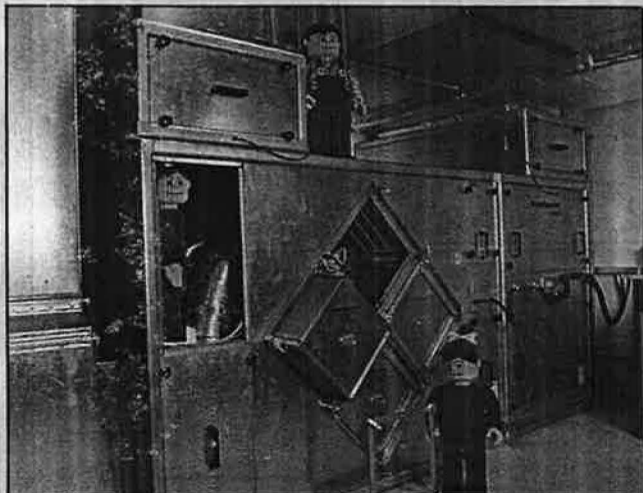
Lego technicians inspect the Dantherm heat-recovery air-handling unit in the model workshop.
