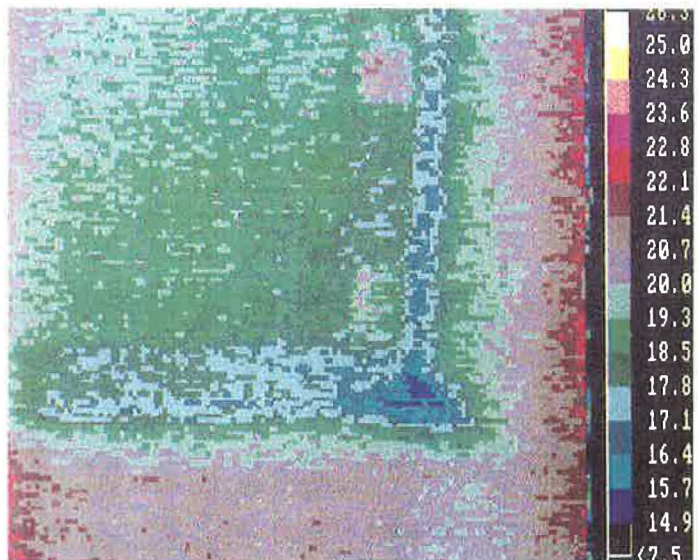
Air leakage (purple/blue) around the window frame is clearly highlighted in this IR thermography scan
