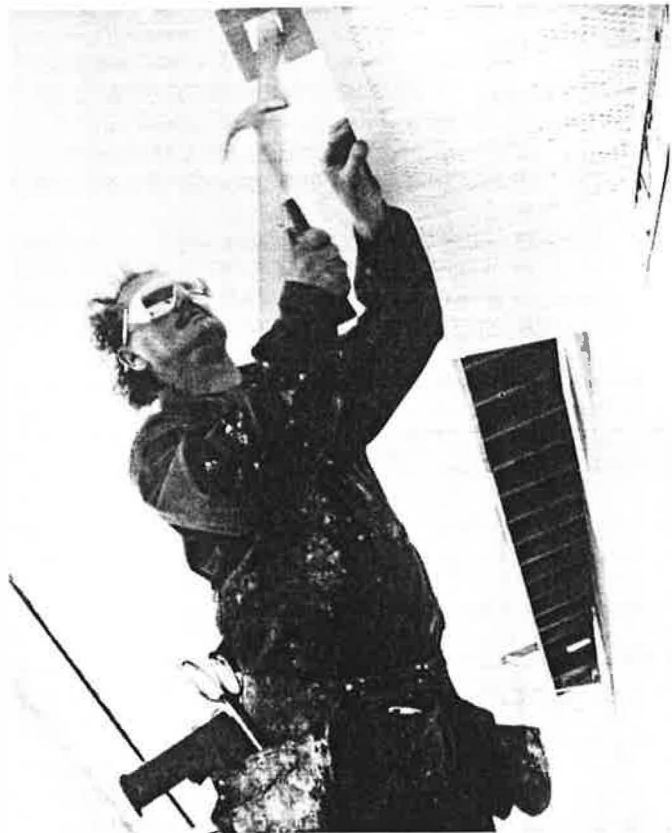
Courtesy of Ontario Hydro
