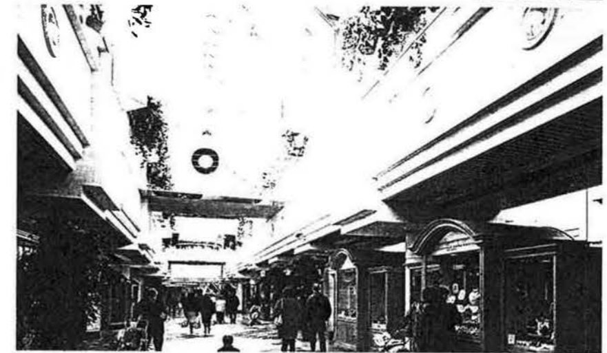
Mr. Searle's company, Airstream Environmental Products, installed a smoke ventilation system in the new Olympia Shopping Centre, East Kilbride.
