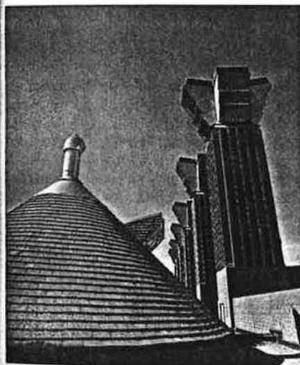
Detail of the amazing roofscape with the natural ventilation chimneys. The louvres conceal motorised dampers controlled by the bems.
