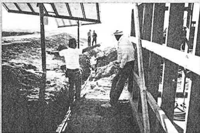
The Idaho Power photovoltaic (PV) program helps customers in remote locations take advantage of a less expensive option for electricity—solar collection. Construction is under way here on a PV array for a water pumping system for a cattle ranch, designed to process over 10,000 gal per day.
