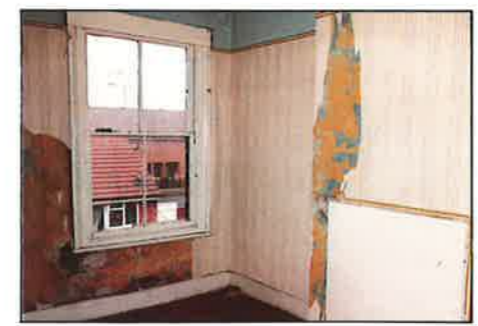
Figure 4. Plaster in need of replacement, room requiring redecoration.
