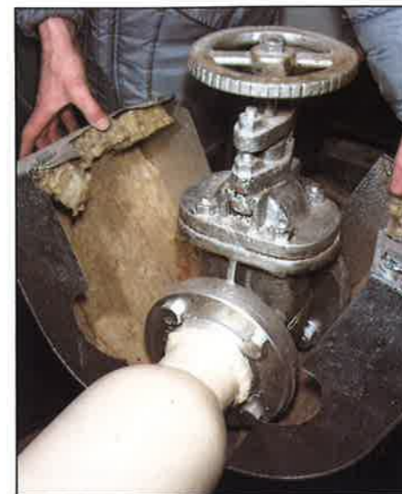
Hither Green School: Boiler House. Insulation of pipework should include flanges
