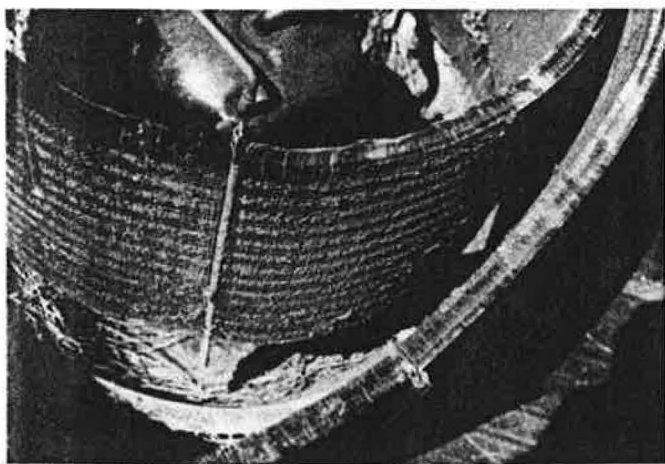
This dirty outdoor coil caused the compressor to "blow."
