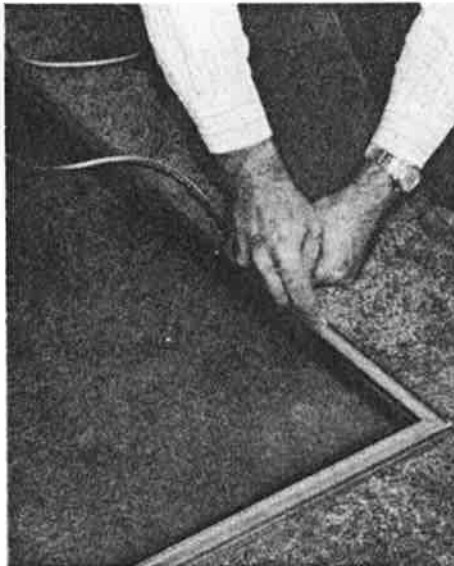
Re-weatherstripping a window using modern pile type material incorporating a plastic film
