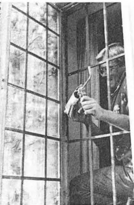
Caulking the static part of a casement window on an historic building
