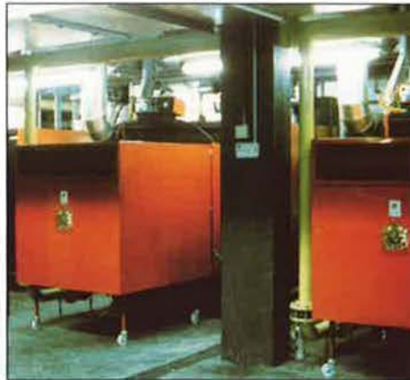
The condensing boilers at Solihull Metropolitan Borough Council.
