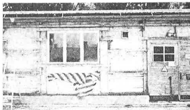
Figure 1 One of the facades of the selected building during the replacement of the insulation in the exterior walls.
