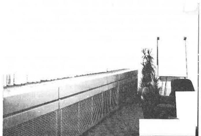
Figure 15 Induction unit for a heat-source ventilation system in a conference room.
