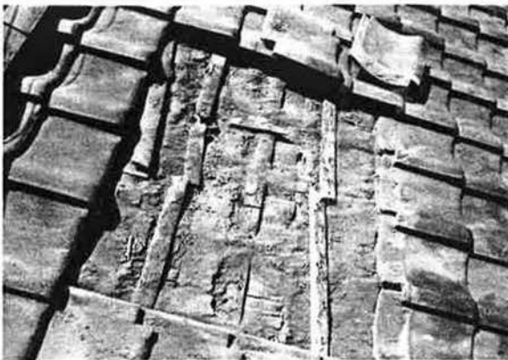
Fig. 12. Ash of 13 172 g/m 2 in weight lying beneath roofing tiles (observed in Tarumizu city, 6.7 km from Sakurajima; house age = 24 years; roof pitch = 40/100; Japanese style of tile).
