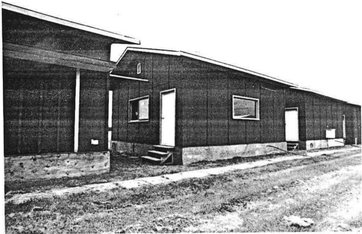
Figure 3-3 Reference Unit 5 from north-east showing plywood sheathing over vapour barrier on concrete basement.
