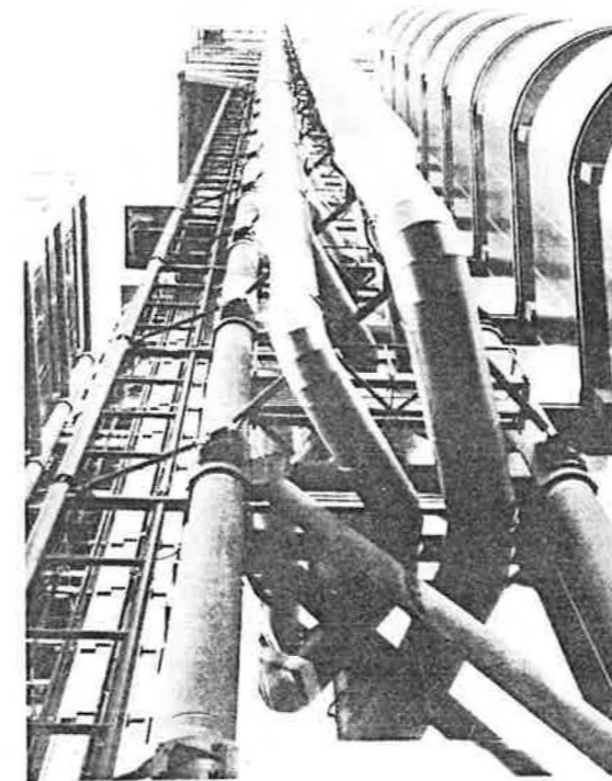
Figure 7.2 Vertical ductwork descending from plantrooms
