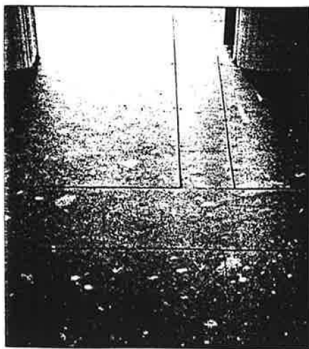
The insulated floor with removable panels to provide access to pipework.
