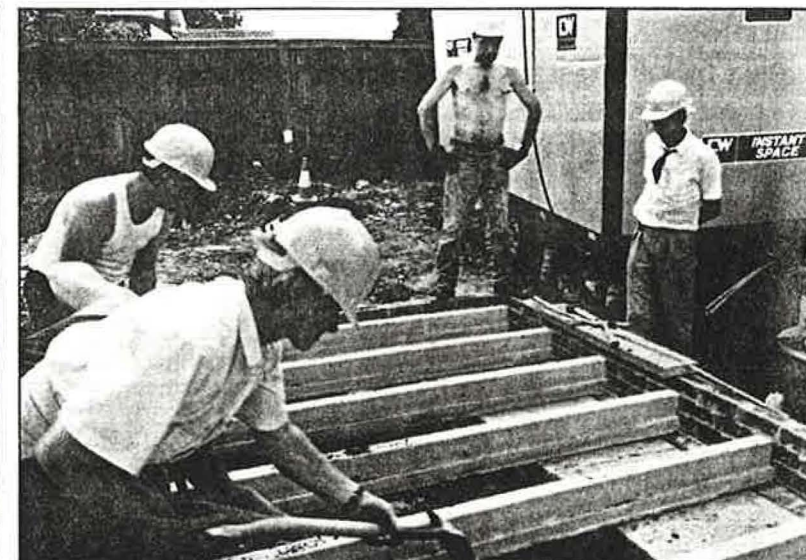
The pot and beam suspended ground floor is insulated on the underside
