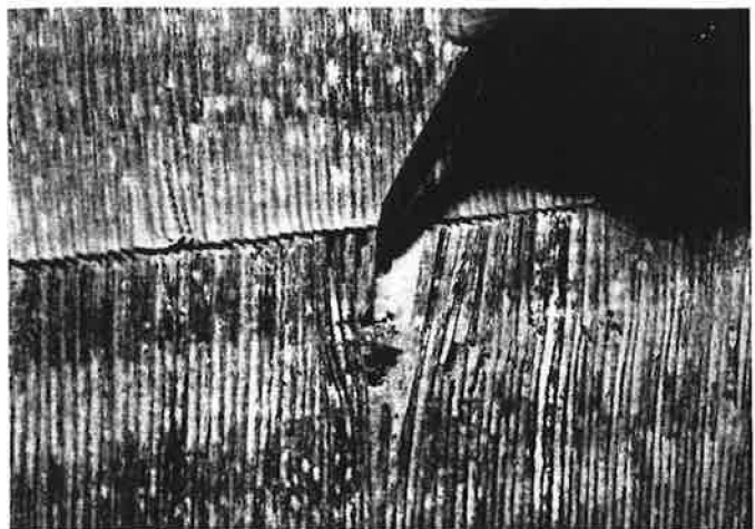
Figure 1 Bimetallic corrosion on the two-year-old dehumidifier coil at pool O 3 -1
