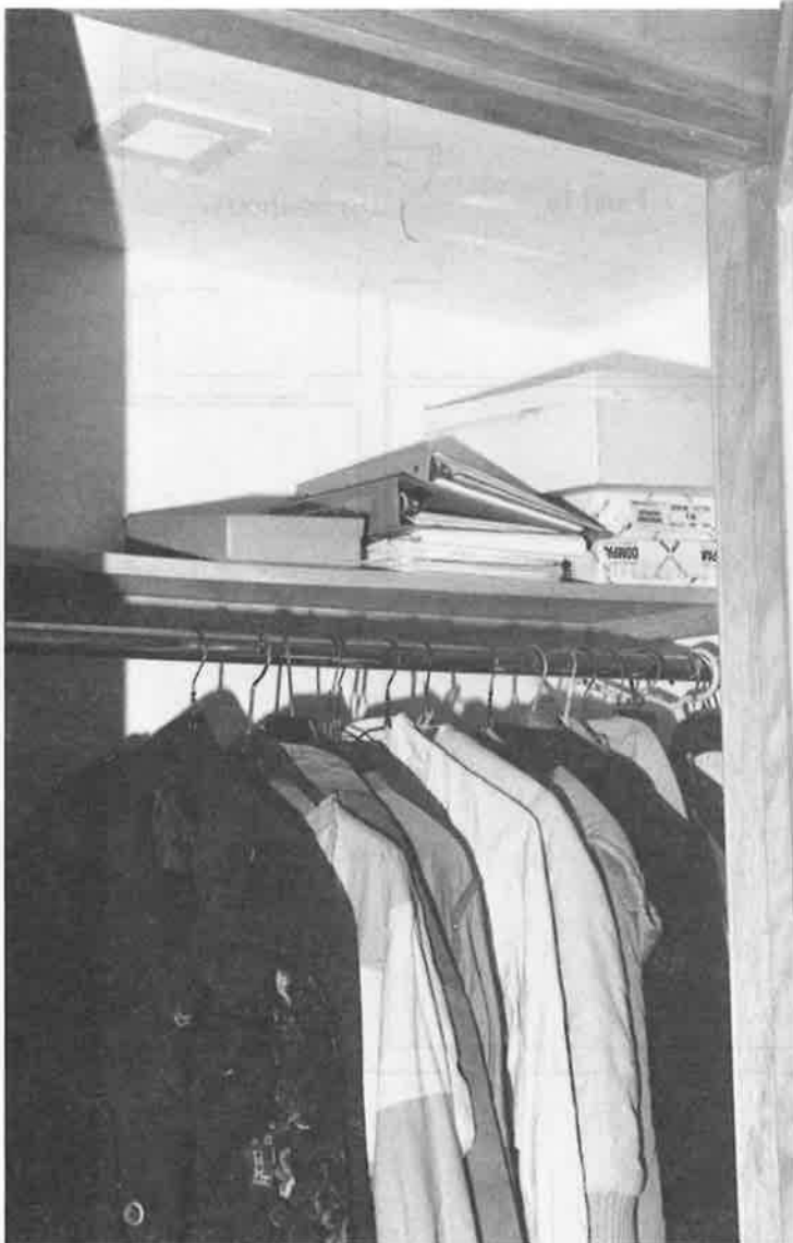
EXHAUST GRILL IN CLOSET CEILING
