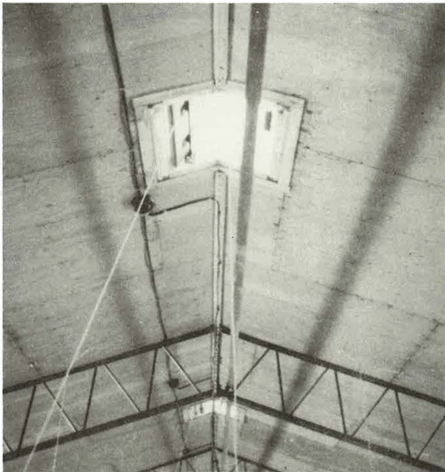
Photo 4 Chimneys with baffle and manual control cable as seen from below. The baffle is in the fully open (summer) position.
