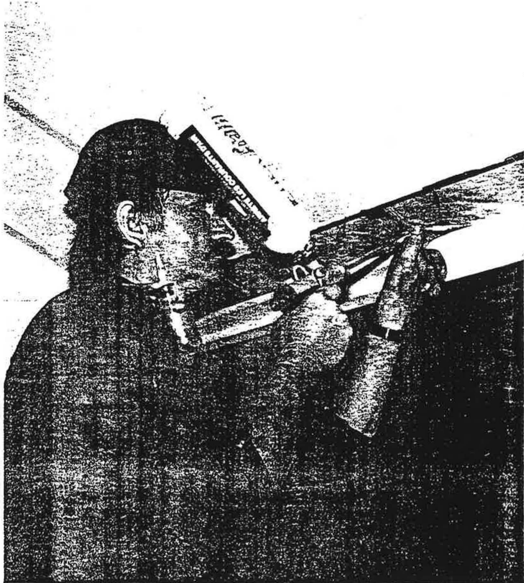
Figure 6 Single component foam being used to seal top of window frame to concrete lintel.
