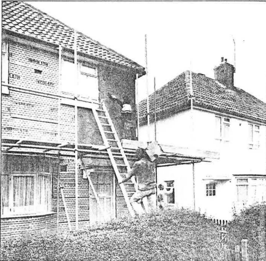
A Harrow house is clad with the Insolath external wall insulation system
