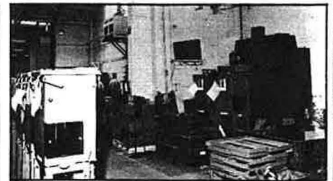
A PGUH heats the workbay and a direct fired warm air heater is used in the assembly area
