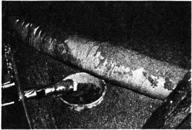
Figure 3. The condensate line in this picture was "plumbed" into a five-gallon bucket filled with rocks and set in the attic. This caused the sheetrock underneath to sag. The condensate line should have been run to a permanent drain at a constant negative slope.
