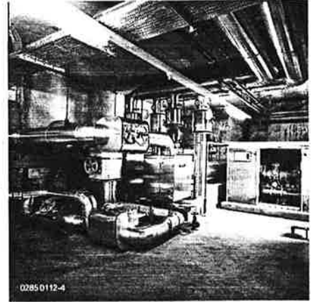
5 District heating infeed with calorifier station. Right: refrigerating machine.
