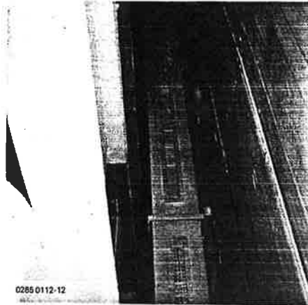
10 Supply air duct at the stage shaft outside wall with air outlet openings directed upward.
