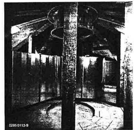
8 Exhaust air duct in the dome above the auditorium, and smoke extraction fan.
