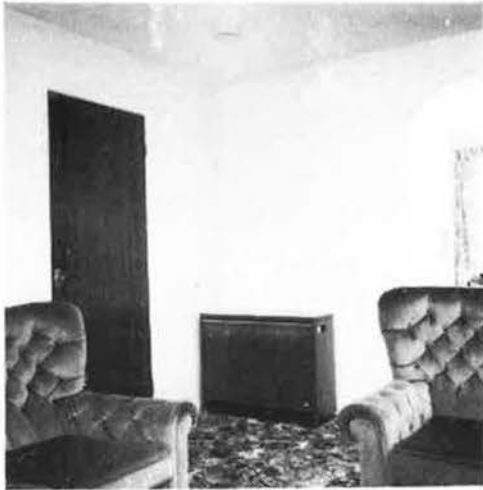
Lounge storage heater
