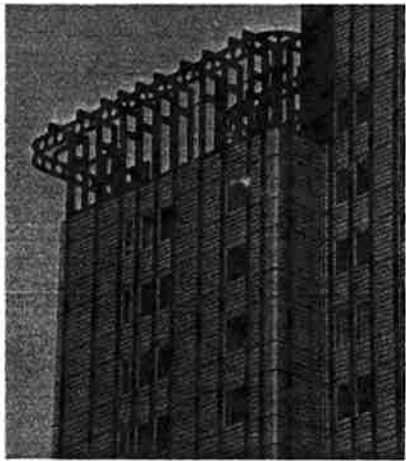
Parson's House overcladding nearly complete (above). Section through new cladding—note ventilation/drainage to cavity (right).
