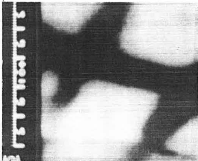
Figure 5.9 Bedroom ceiling seen from below shows cold patches under joists and missing insulation patch.
