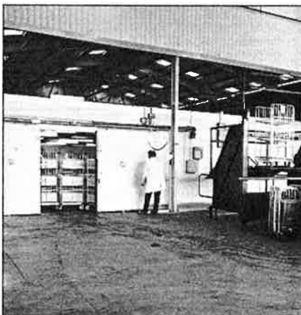
Fermatic sliding door track in use at the new Job's Dairy warehouse complex
