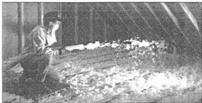
Figure 3 — Flat ceilings in the Millennium Home were blown with 18.5 inches of loose-fill fiberglass (R-50); vaulted ceiling have R-38 batts.
