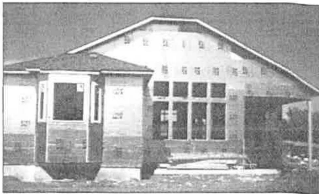
Figure 2 — A&S Homes is pioneering the use of insulating sheathing (1" polyisocyanurate) in Manitoba, Canada. The 6-inch wall cavity behind the sheathing is filled with batts, yielding an R-27 wall.
