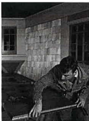
Carpenter Jesse Amar installs a bottom sweep that hides in a channel to seal a major weather gap. This weather strip is almost invisible on old-house doors.
