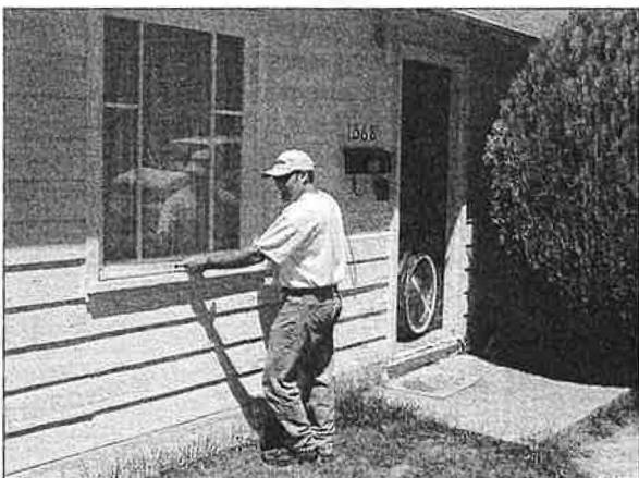
This weatherization technician uses a blower door to identify and treat air infiltration in a Utah home.
