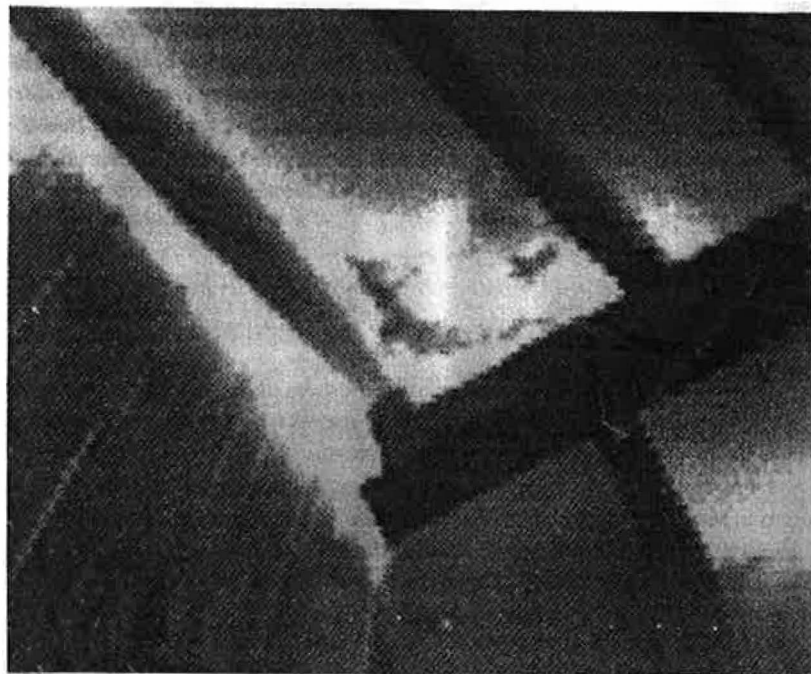
Figure 1 Photograph and thermogram taken within a freezer looking up at its roof in a corner. Frost and ice are present there due to infiltration of warm, moist outdoor air where the two walls and roof join. Airtight seals are needed at such roof-wall intersections.
