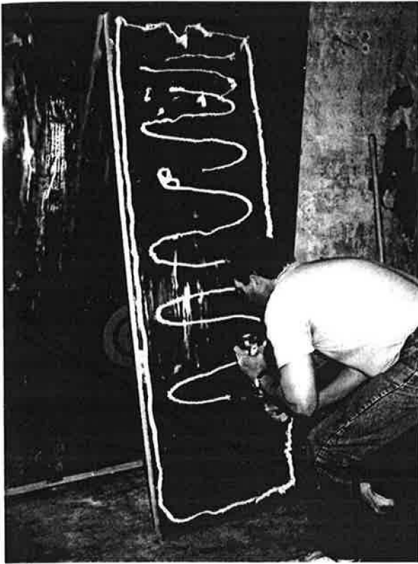
Figure 4 Polyurethane foam adhesive was used to fasten 1½ in. thick rigid foam insulation to the interior surface of the walls. The exterior wall insulation used was a polyisocyanurate insulation with foil facers and an R-12 rating (1½ in. thick). Foam adhesive and drywall screws fasten the ½ in. thick cellulose-reinforced gypsum wallboard to previously installed 2 × 2 wood nailers (top and bottom) and to the rigid foam insulation.
