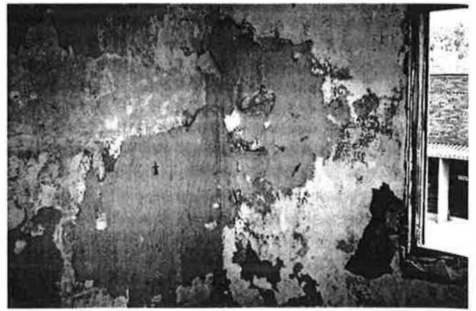
Figure 3 A Public Housing Authority unit was rehabilitated with the installation of an innovative composite wall system. This system undid years of hard use followed by extended vacancy and major moisture damage. High moisture levels from a leaky steam heating system had combined with uninsulated masonry walls to destroy the exterior wall lath and plaster finish.
